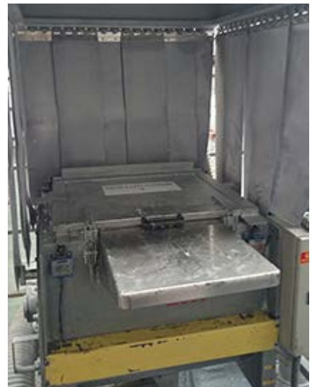
Plastic curtains installed in the areas immediately surrounding local ventilation systems to help increase the efficiency of operating spaces around the section where raw materials are inserted into each system
