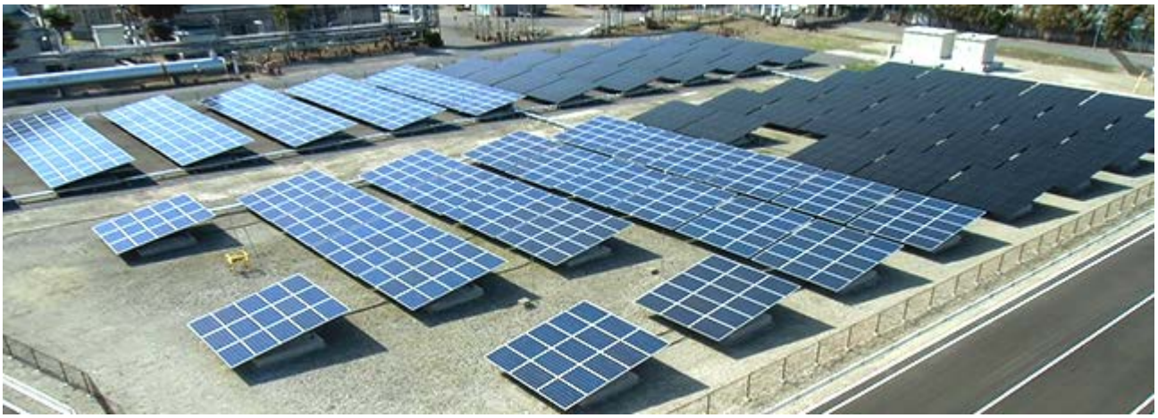
The testing facility and demonstration power plant within its Mobara Branch Factory site
