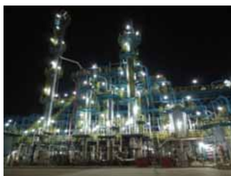
(Left) EPT Plant
