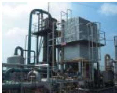
Exhaust combustion facility
