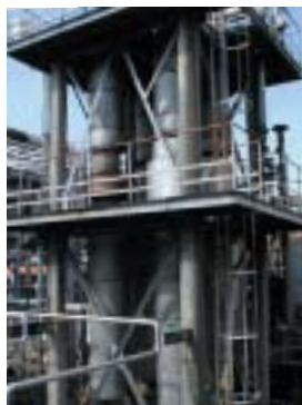
Wet-type oxidation facility
