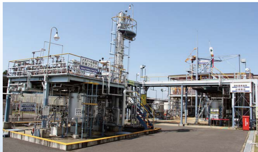
Methanol distillation training plant and water operation facilities
